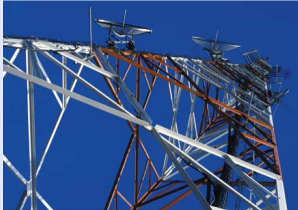
Sentor is a complete Tower Site Automation and Control System
